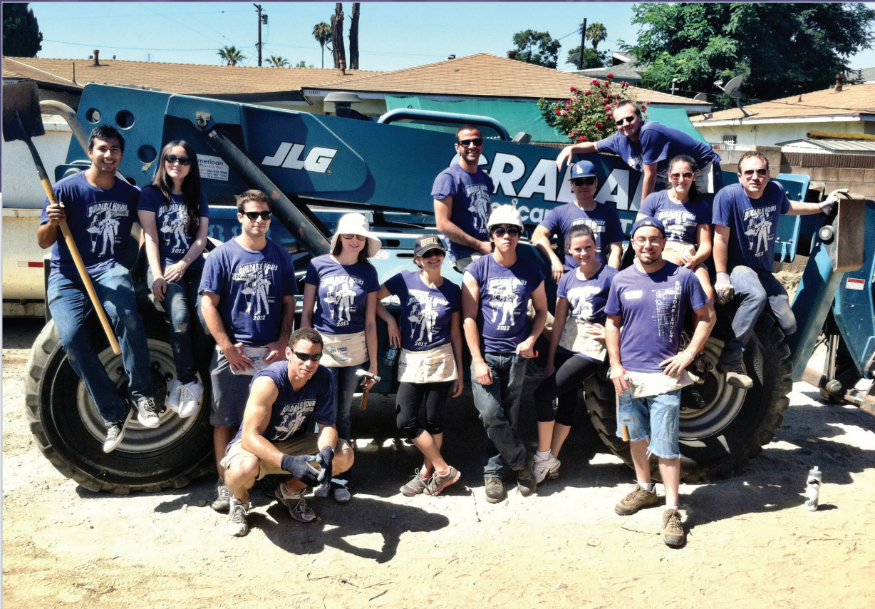
Summer associates and staff from the Los Angeles area help build a home for a family of three on a Habitat for Humanity of Greater Los Angeles site.
